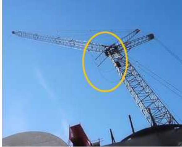
Jib stops are required on tower cranes.
